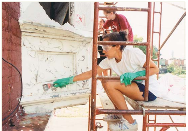
Students from Rowan University working on a house for Habitat for Humanity. Photo courtesy Rowan University.
